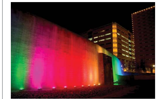
Infrastructure Lighting Installations
